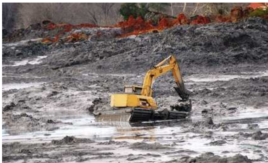
A trackhoe scoops up spilled coal ash which is being loaded into rail cars for shipment to an Alabama landfill in Perry County for disposal. (Special/TVA)
