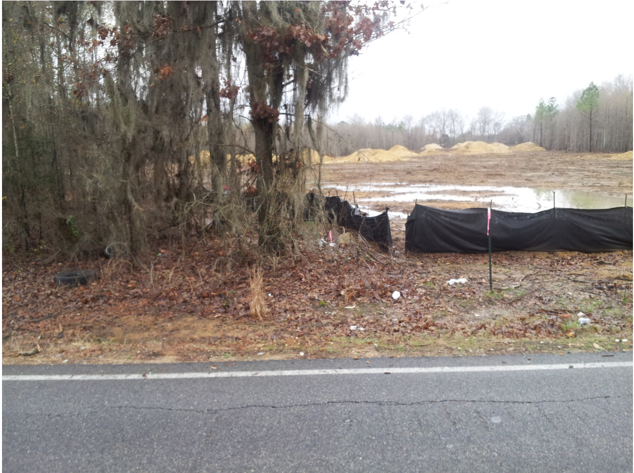
Failure to Maintain Silt Fences 12.23.2013
