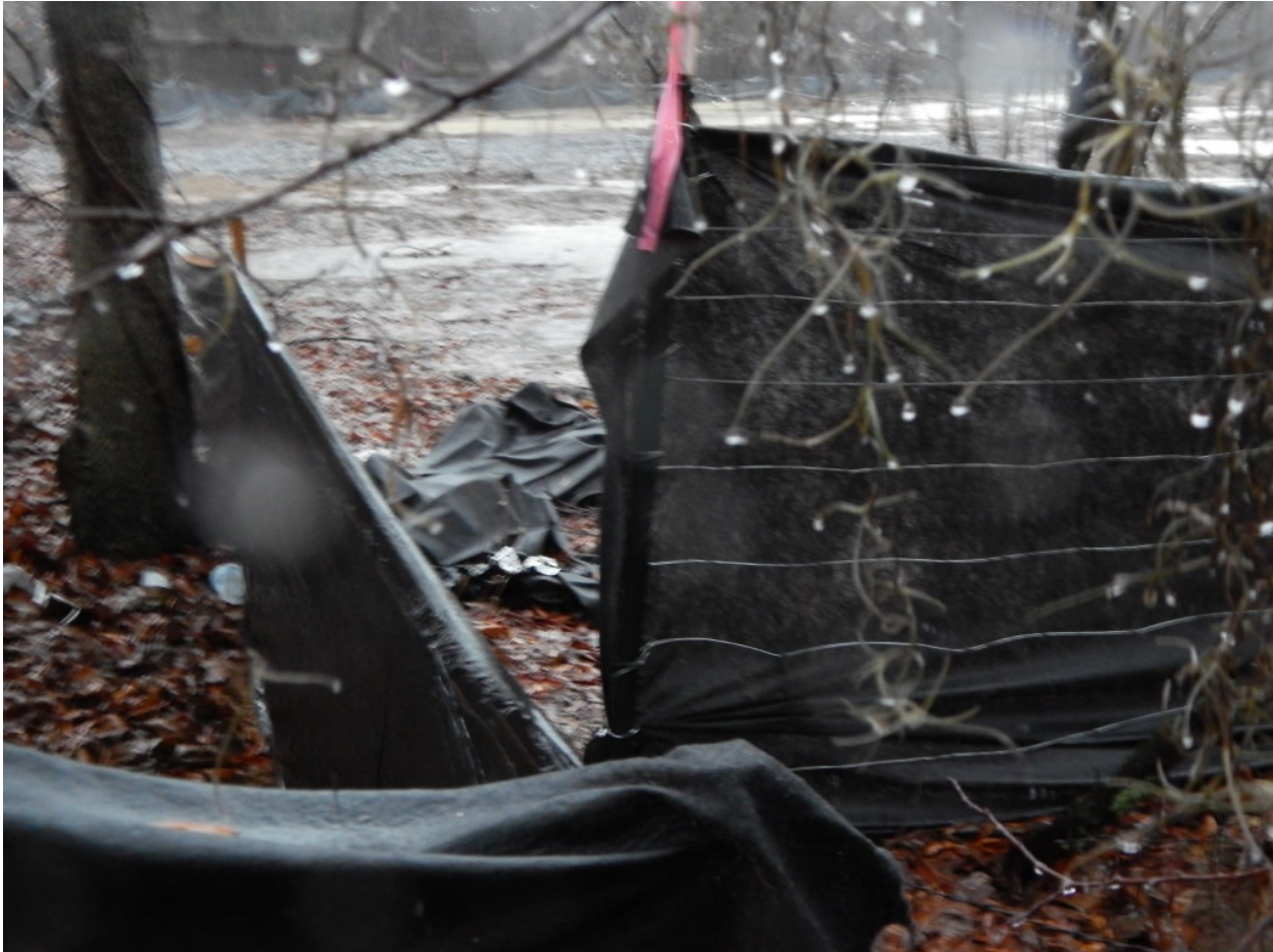
Failure to Maintain Silt Fences 12.28.2013
