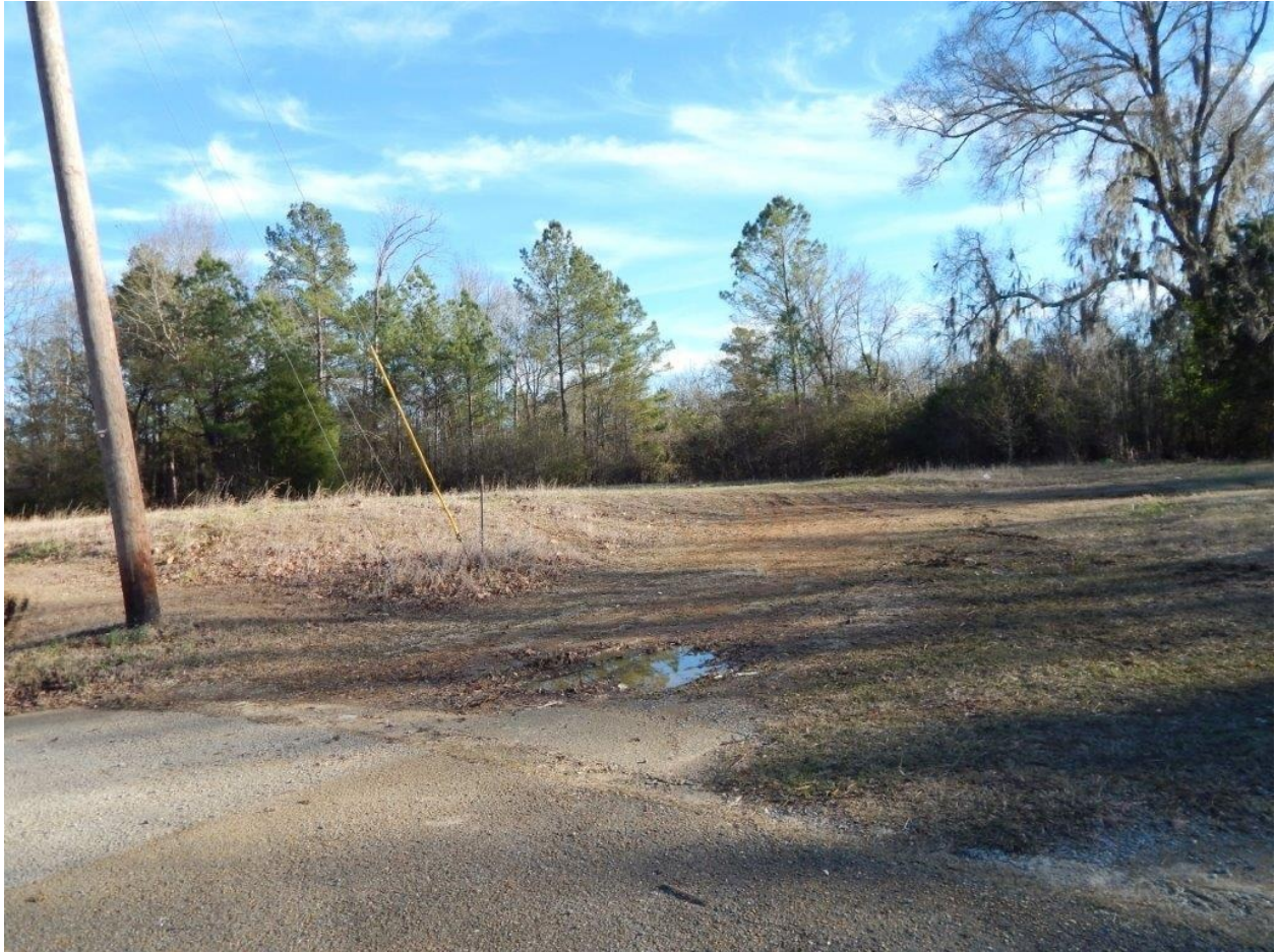
Failure to Stabilize Andova Drive Entrance/Exit 11.18.2013
