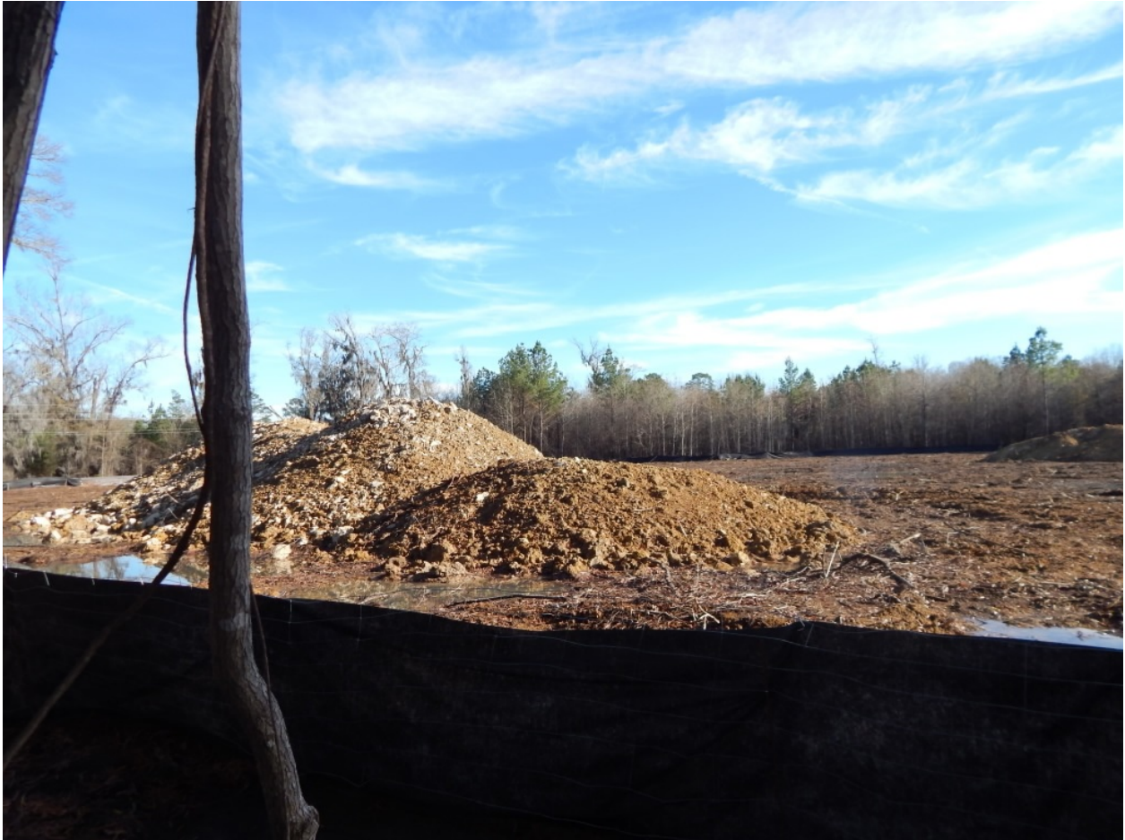
Failure to Provide Temporary Stabilization 1.3.2014
