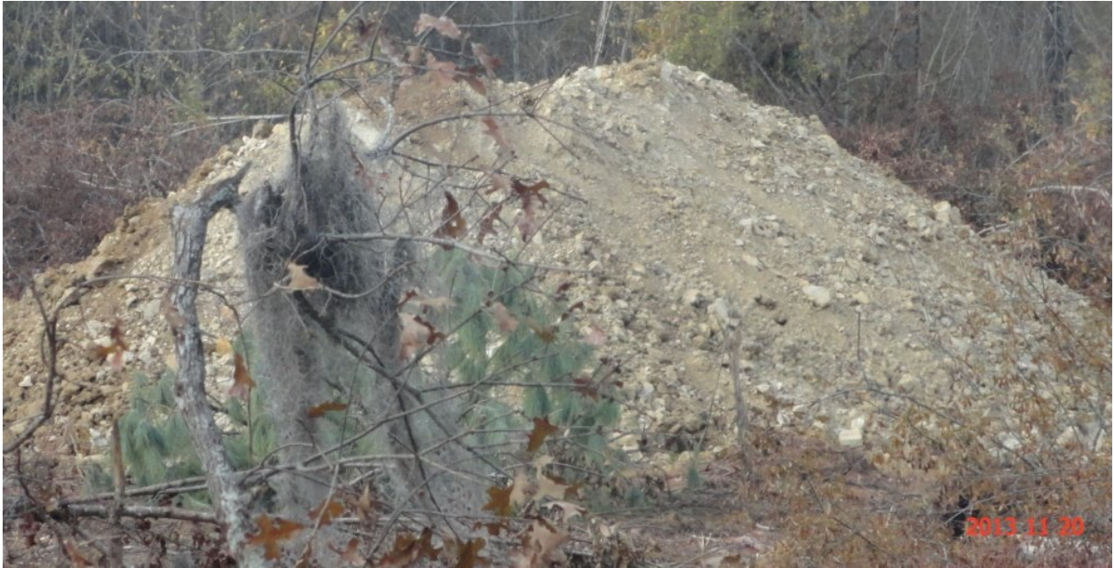
Failure to Provide Temporary Stabilization 11.20.2013
