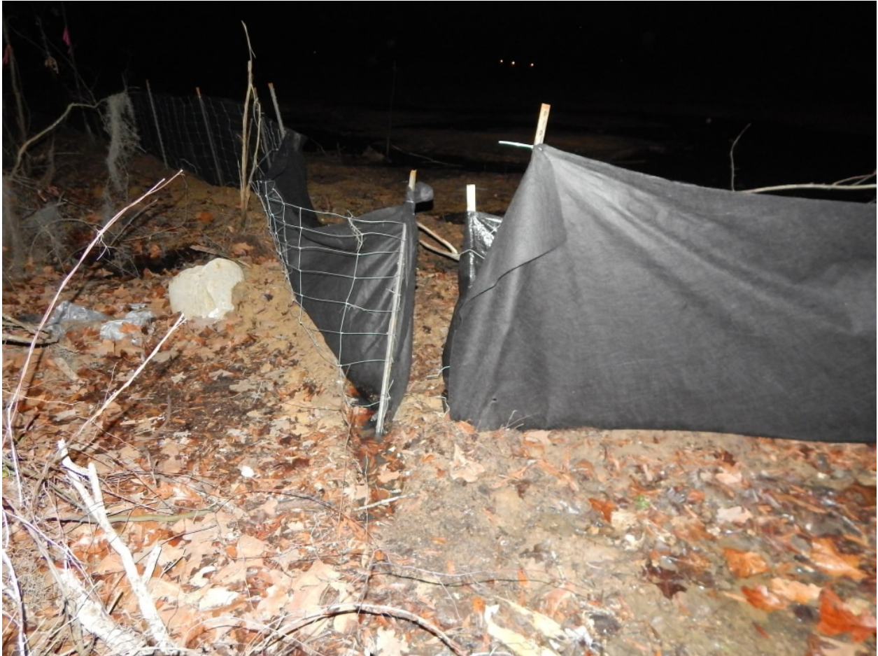
Failure to Maintain Silt Fences 1.2.2014
