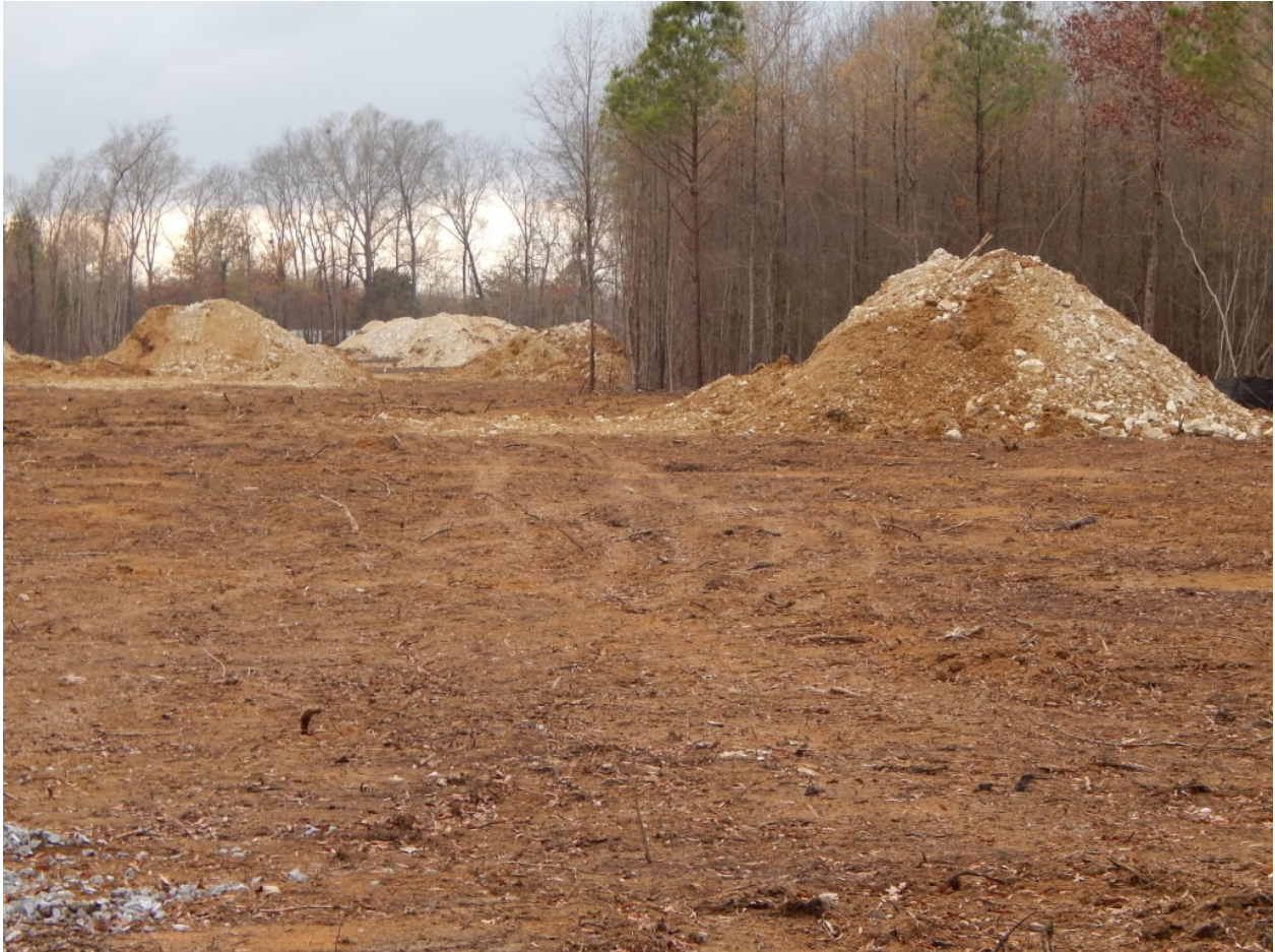
Failure to Provide Temporary Stabilization 12.21.2013
