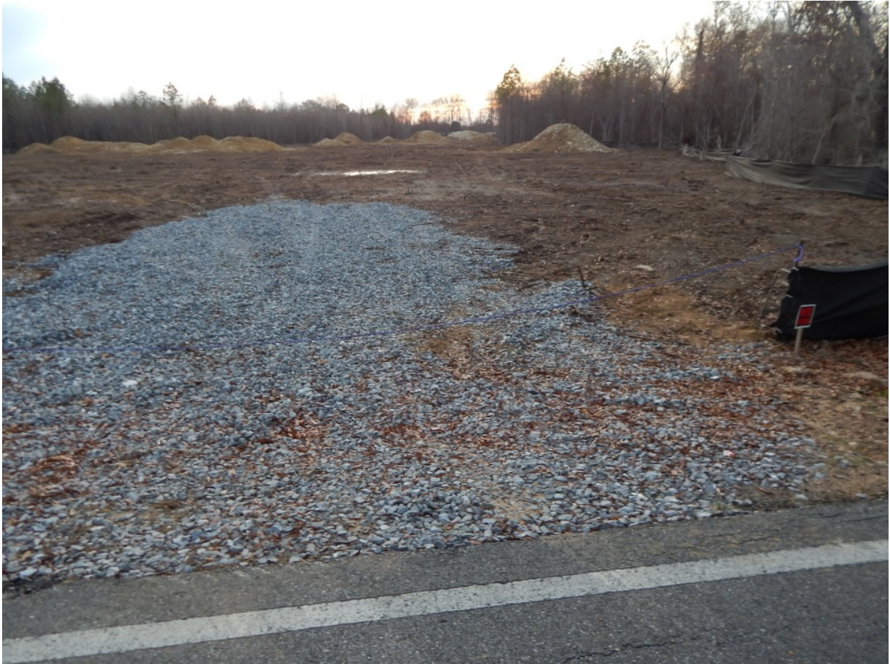
Failure to Stabilize Woodley Road Entrance/Exit 12.26.2013
