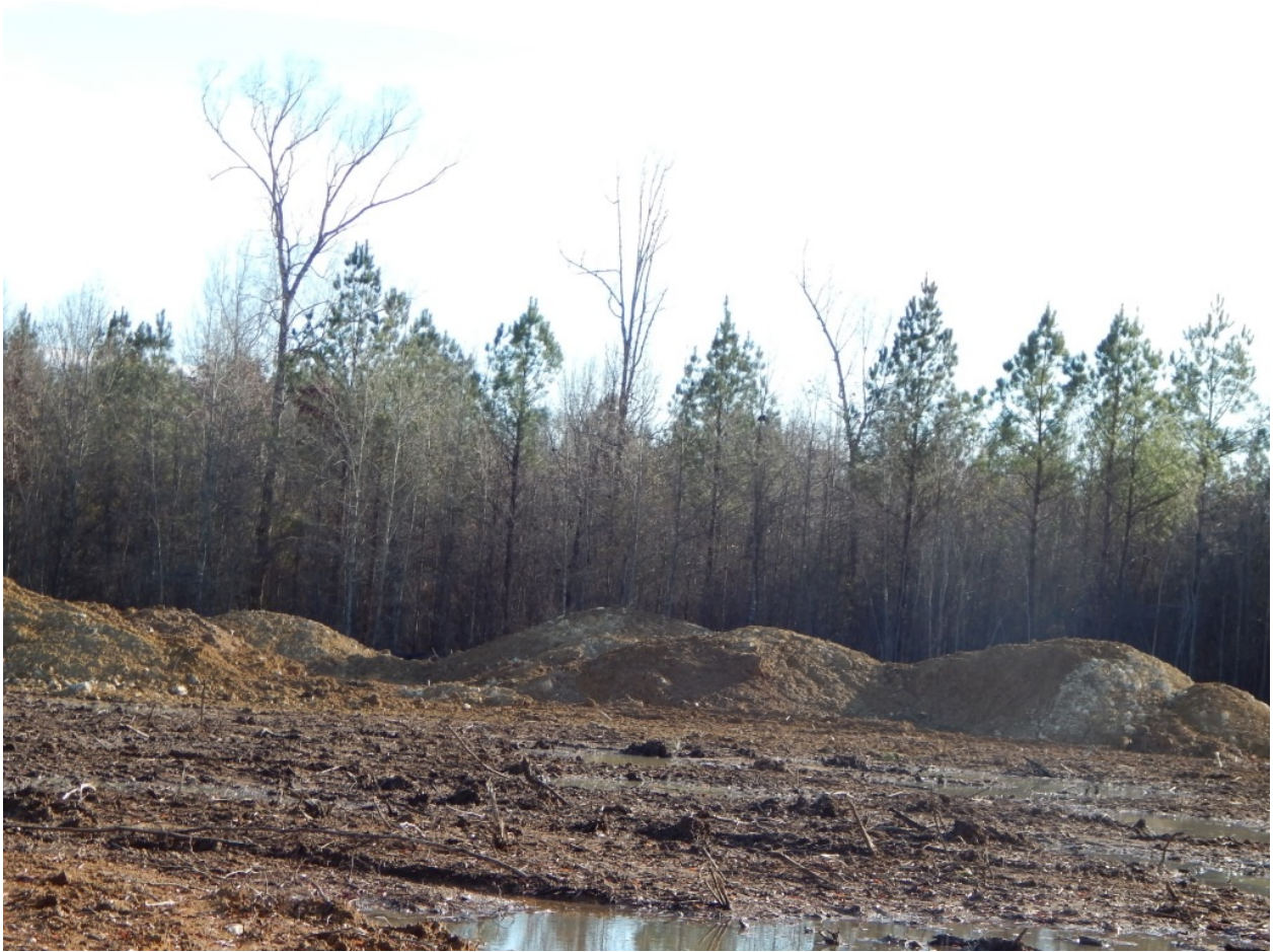
Failure to Provide Temporary Stabilization 1.3.2014
