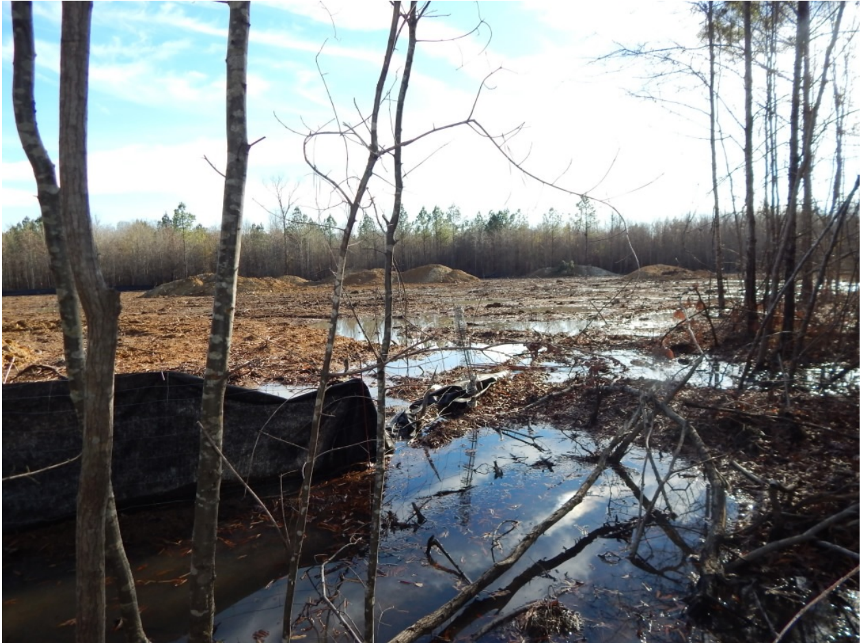
Failure to Implement/Install Sediment Control Measures
