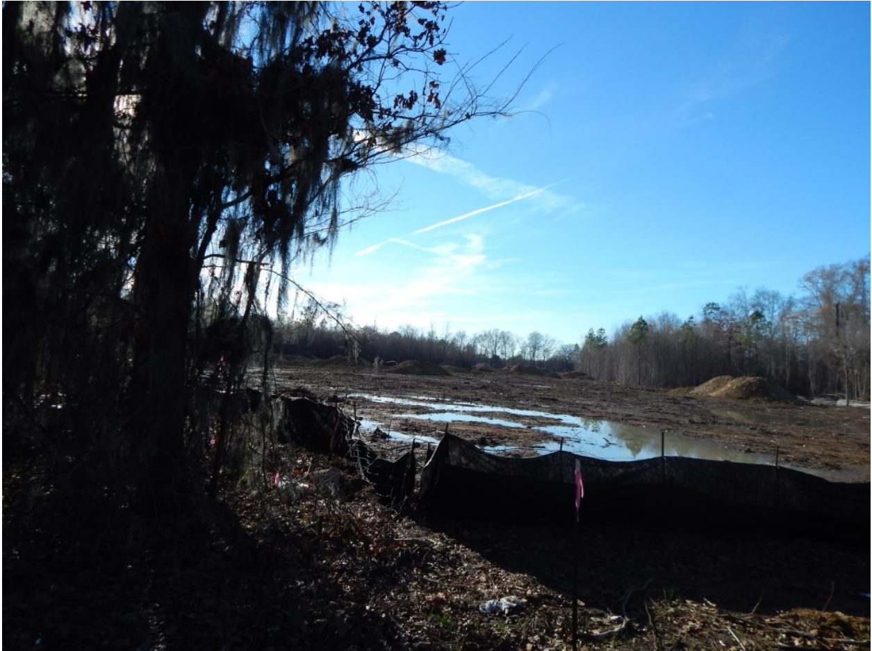
Failure to Maintain Silt Fences 1.3.2014
