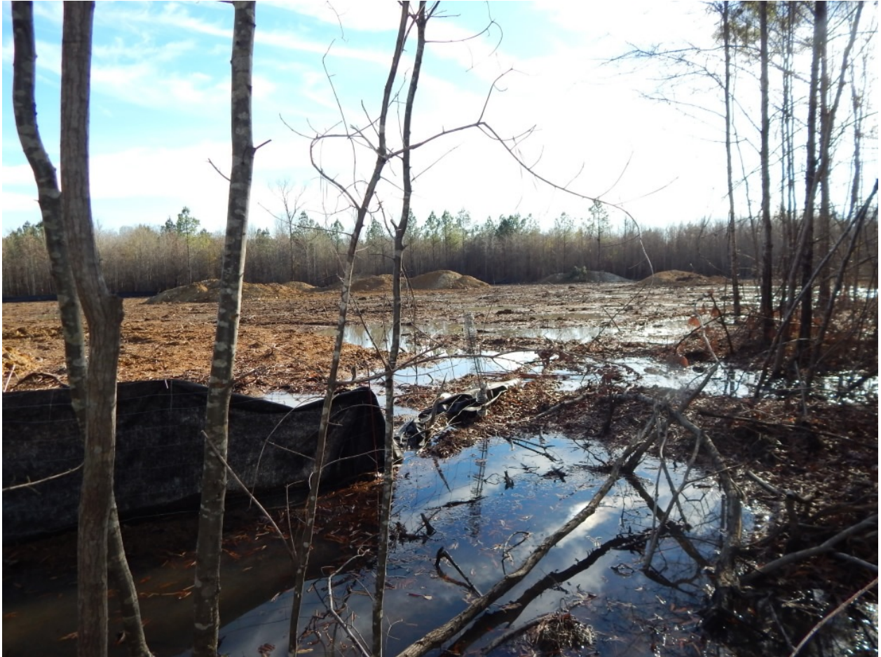
Failure to Provide Temporary Stabilization 1.3.2014
