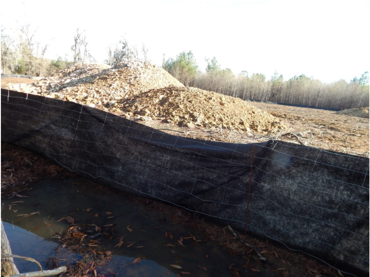
Failure to Provide Temporary Stabilization 1.3.2014
