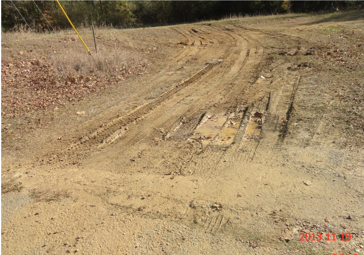
Failure to Stabilize Andova Drive Entrance/Exit 11.19.2013
