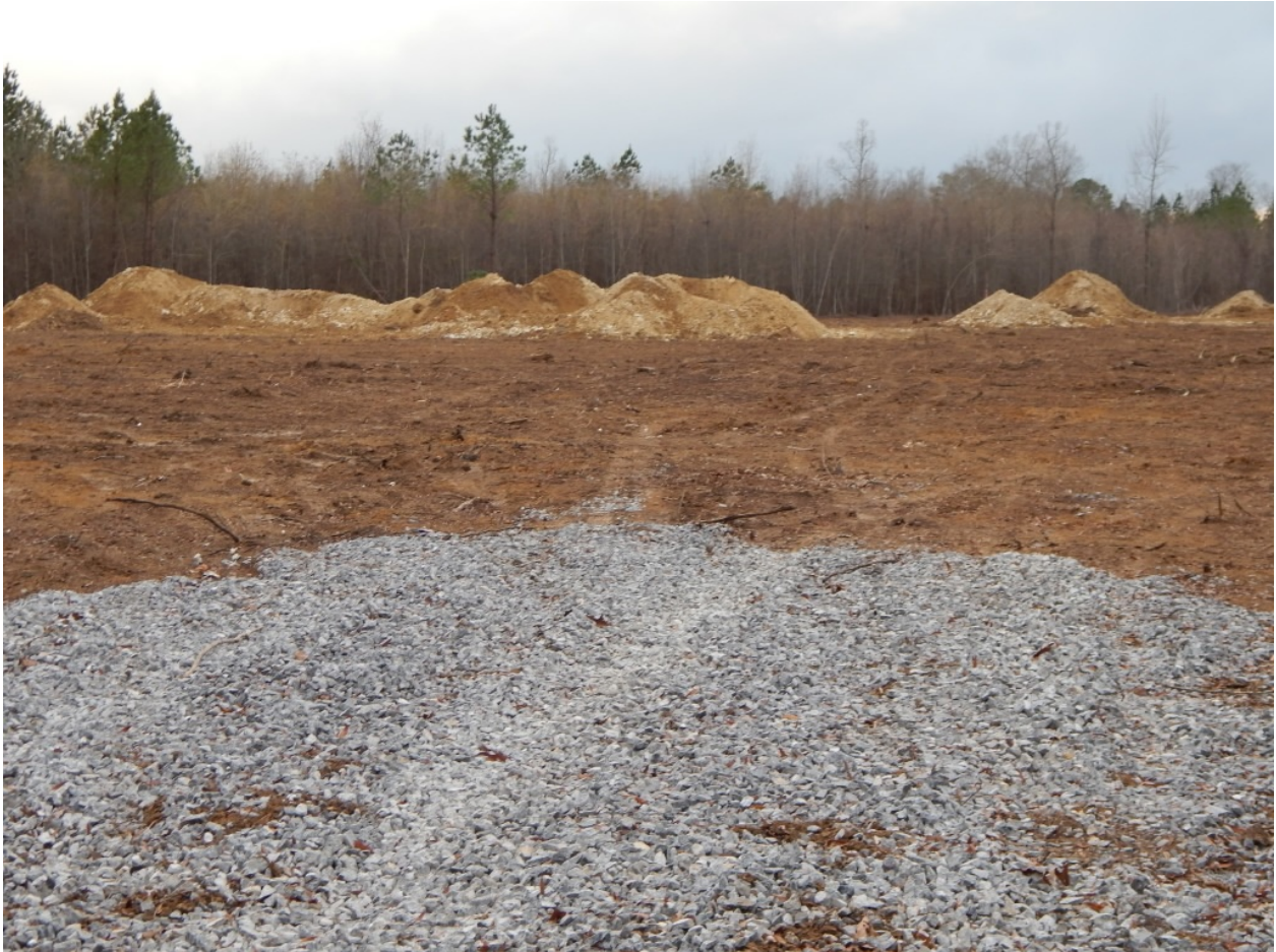
Failure to Provide Temporary Stabilization 12.21.2013
