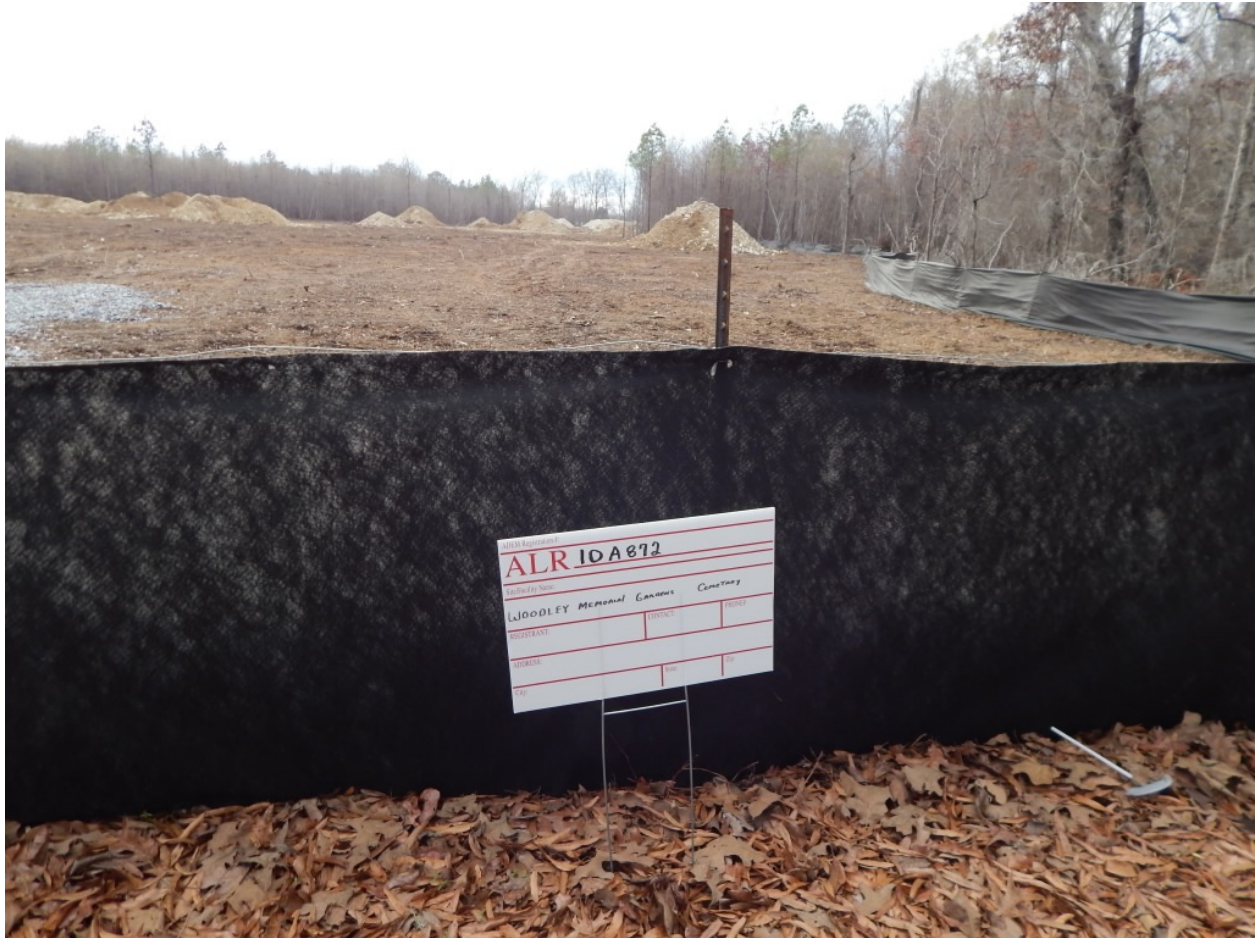
Failure to Provide Temporary Stabilization 12.21.2013
