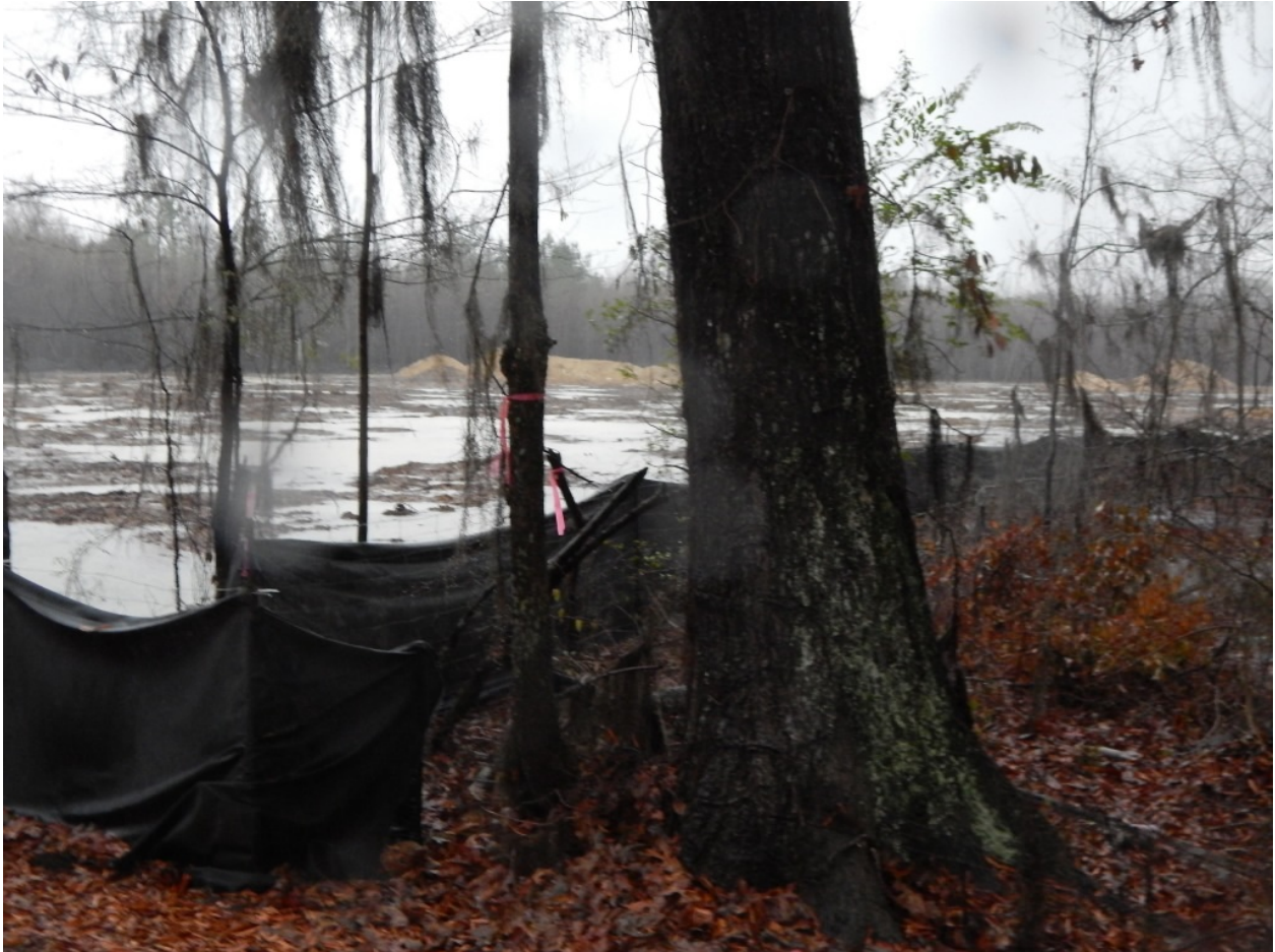
Failure to Maintain Silt Fences 12.28.2013
