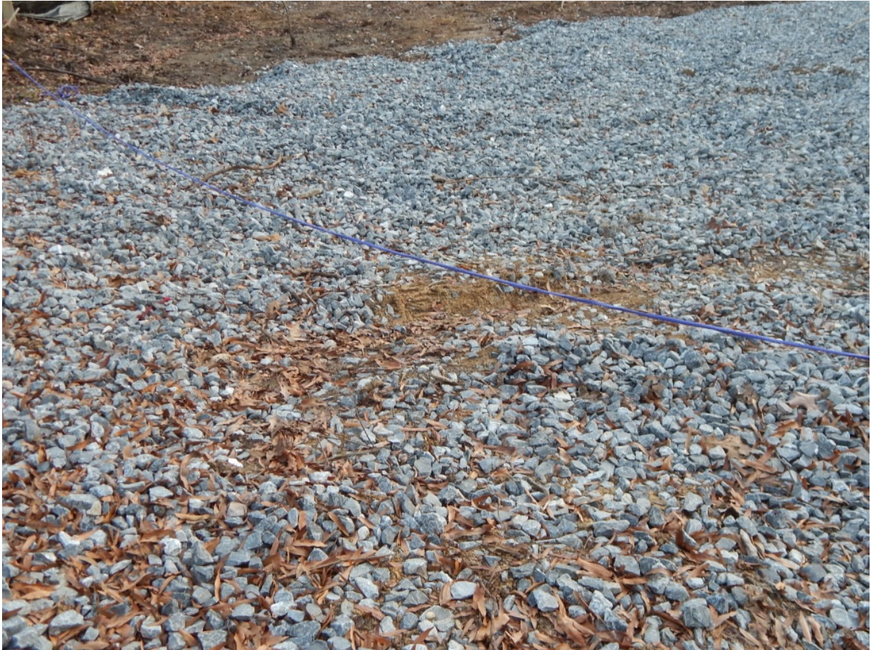
Failure to Stabilize Woodley Road Entrance/Exit 12.26.2013
